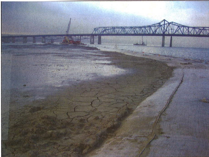
Backfilling the artificial island after establishing the geocontainer-secured perimeter. Photo by Maccaferri.
